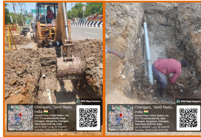
140mm PVC pipe line leak was rectified and water supply effected on 19.05.2026 under CWSS to Chengam,Pudupalayam TPs and 40 wayside habitations in Chengam,Pudupalayam unions in Thiruvannamalai district
