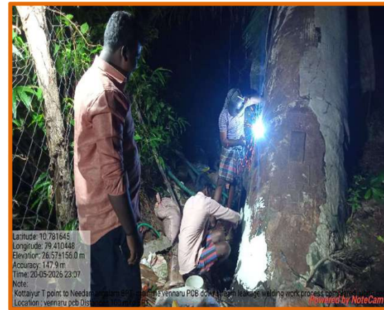
1100 mm MS pipe line leak was rectified and water supply effected on 20.05.2026 under Vedaranyam CWSS in Thiruvavur district
