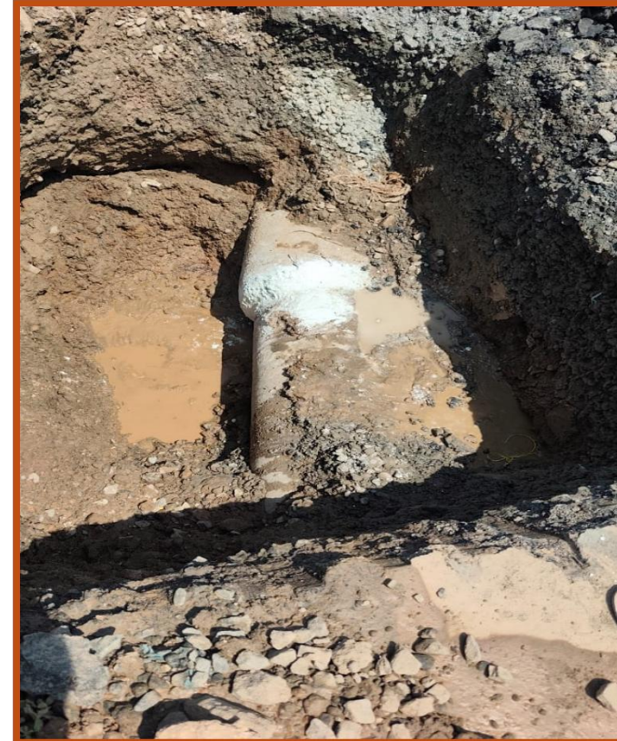
Damaged 450mm DI Pipe leak was rectified and water supply effected on 01.06.2026 under Aravakuruchi CWSS in Karur district
